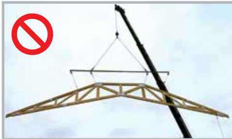
Spreader Bar is too short for this truss.
